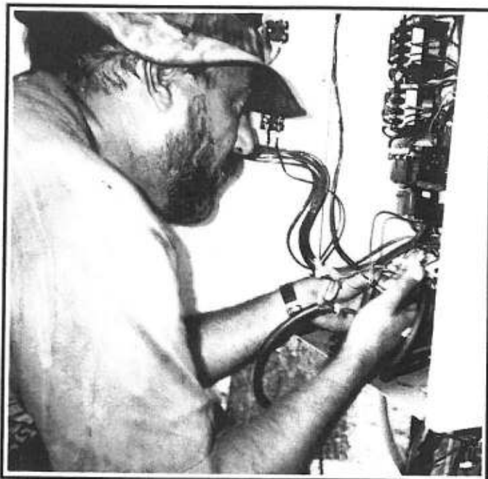
Grizzly wires pump station for the camps sanitation system
